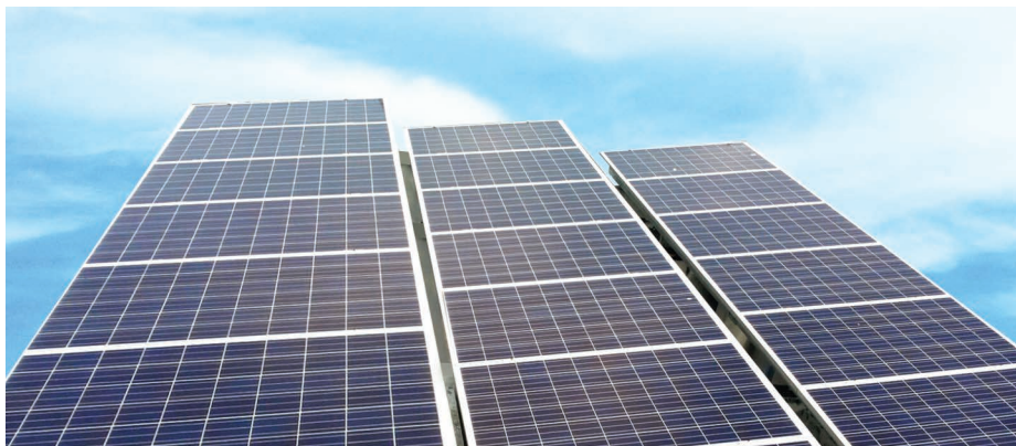
Solar Panels at Narahenpita Branch
